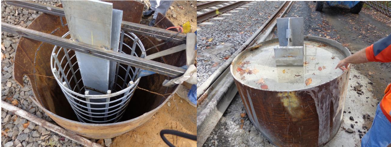
Figure 1. Catenary Hole Drilled and Set with Rebar (left) and Hole Filled with Concrete (right)
