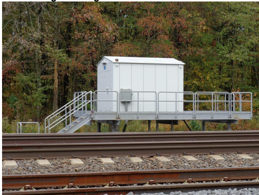
Figure 2. Signal Hut on Raised Platform
